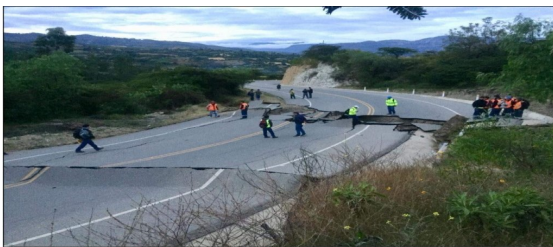
Image: Road damage in Peru Source: temblor.net
