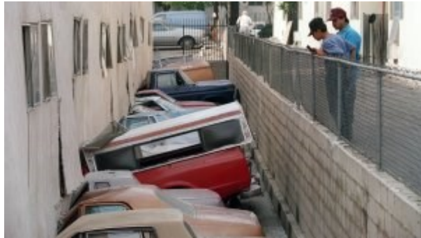
Image: Soft story apartment complex in L.A after Northridge Source: A. CLARY/AFP/Getty Images
