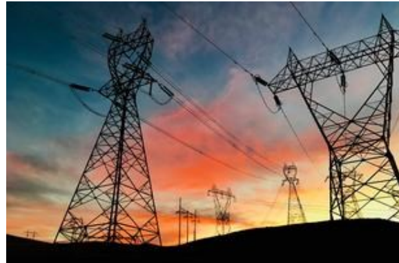
Image: Power grid of Bonneville Power Administration in Oregon.
