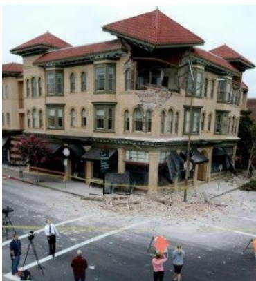
Image: Collapse of Alexandria Building after 2014 South Napa earthquake.
